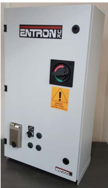
Example: Complete EN7000 system.
